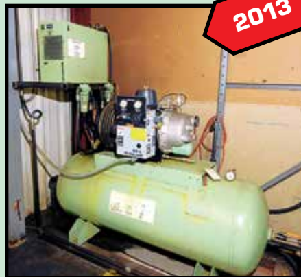
SULLAIR ROTARY SCREW AIR COMPRESSOR AND DRYER
