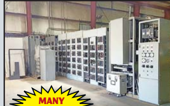
VIEW OF MOTOR CONTROL CENTER
