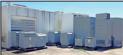
VIEW OF TRANSFORMERS
