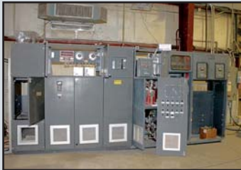
VFD AND SCR LINEUP GEAR
