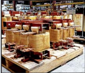
CLOSE UP VIEW OF REACTORS
