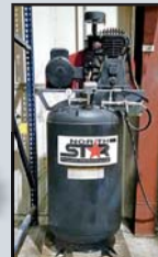
NORTH STAR COMPRESSOR
