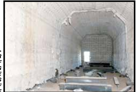
> INTERIOR VIEW OF ROLLING FRAME STRESS RELIEF FURNACE
