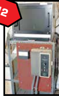
VIEW OF SCHENCK RETROFITTED CONTROL
