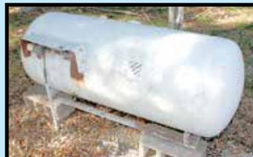
PROPANE STORAGE TANK
