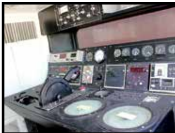
TEST STAND CONTROL PANEL
