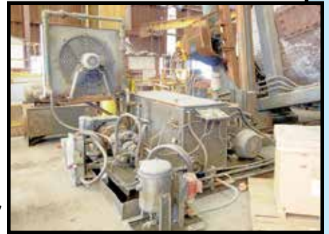
HYDRAULIC SYSTEM OF MDY ENGINEERING CORPORATION ROTARY HEARTH FURNACE
