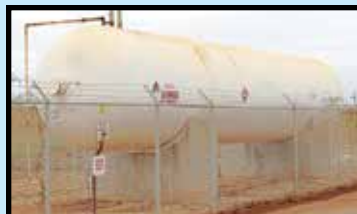
15,000 GAL. CAP. LPG STORAGE TANK
