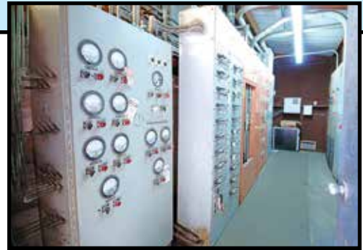
DUST COLLECTOR MOTOR CONTROL CENTER
