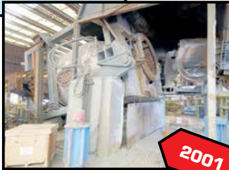
MDY ENGINEERING CORPORATION ROTARY HEARTH FURNACE
