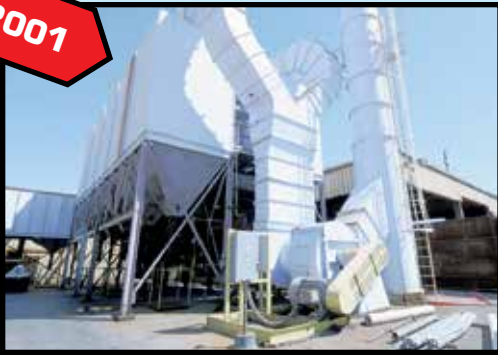
BAGHOUSE DUST COLLECTOR
