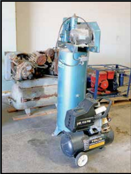
ASSORTED AIR COMPRESSORS
