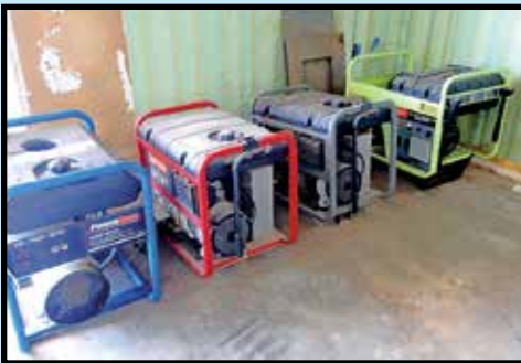
VIEW OF GASOLINE GENERATORS
