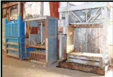
PARTIAL VIEW OF BALERS
